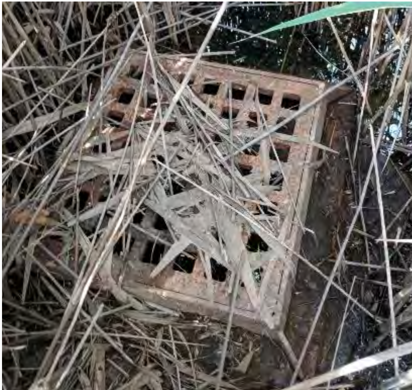
Figure 16. Clogged Outlet Pipe
