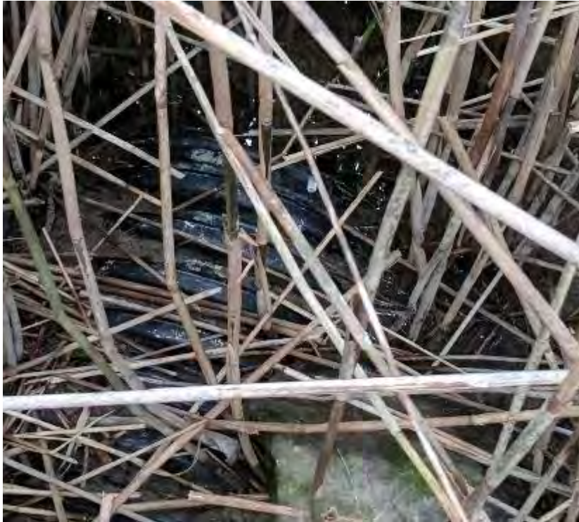
Figure 15. Clogged Inlet Pipe
