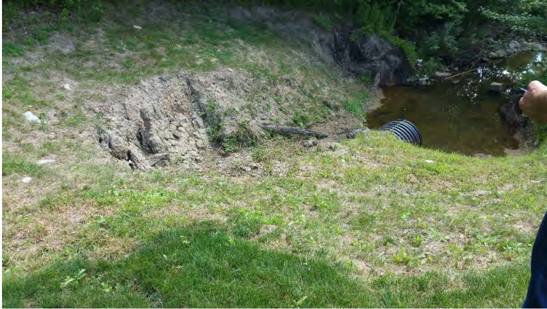
Figure 2. 07-23-2015 photo of erosion between North Point and the Dales.
