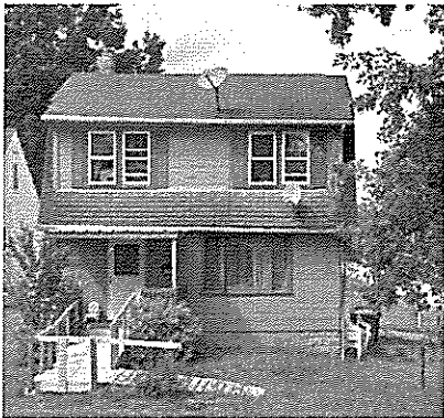
1207 Portage Trail – Constructed in 1952, this residential structure has peeling paint, an older roof, and a dilapidated handicap ramp.
