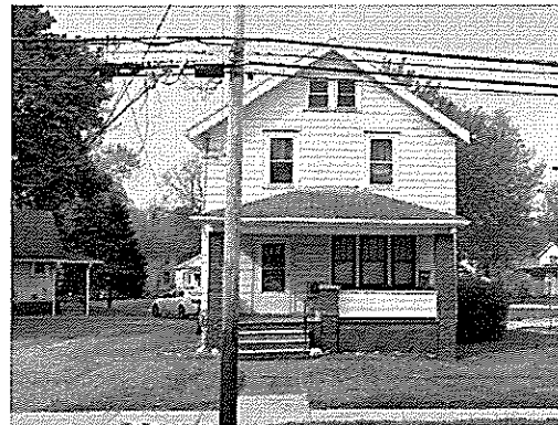
706 Portage Trail -- Constructed in 1942, this housing unit has original windows and doors with sills and casings that are in disrepair. Front steps are also in poor condition.
